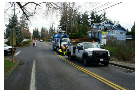
Paving projects were underway this month, as crews ensure city streets are well-maintained.
