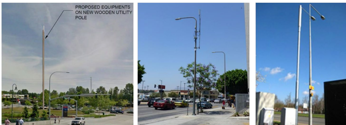
Examples of a poorly designed small cell facility
